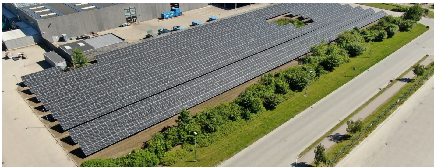
Solar panels at FK Distribution in Taastrup
